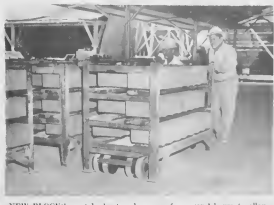
NEW BLOCKS must be kept under cover for several hours to allow them to set up. As soon as a pallet has been filled it is moved from the press to storage (above).
